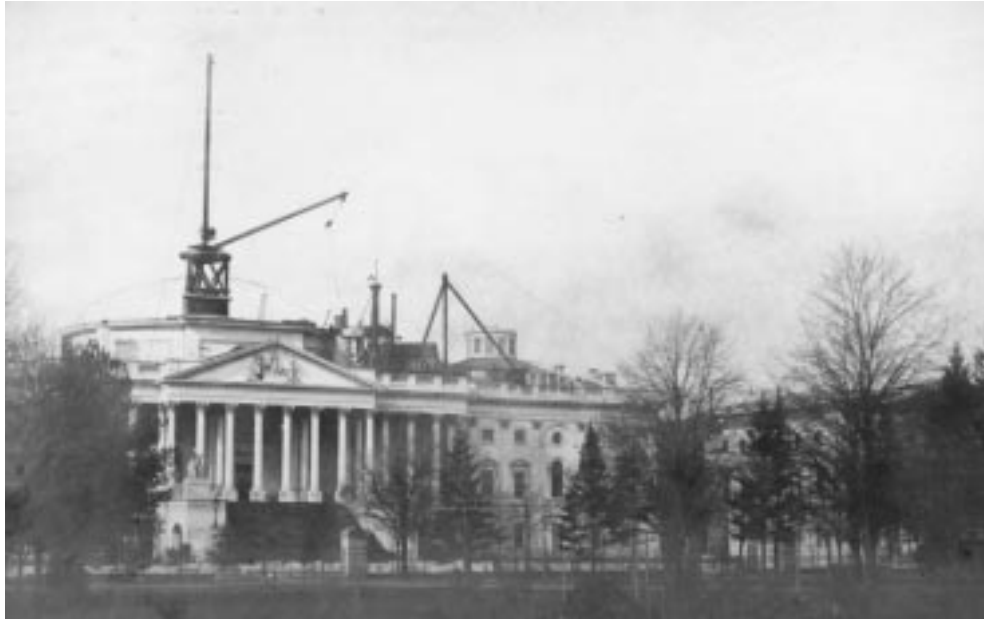
FIG. 8. Photograph of the Capitol dome under construction, with a column lifted to the side. (Courtesy Office of Architect of the Capitol.)
